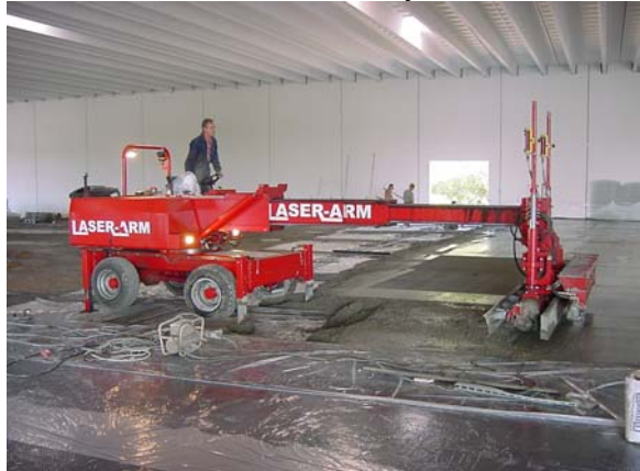
Laser-Arm machine on "pillar floor"
